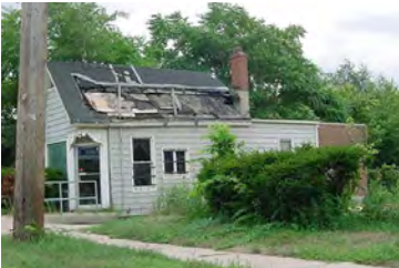
Many residential properties need to be brought up to code.
