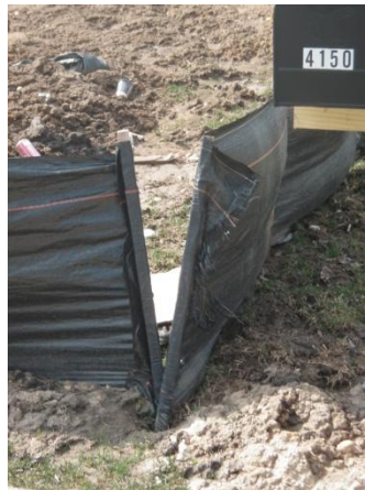
Improper silt fence splice
