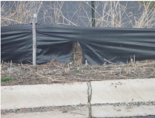
Worn out silt fence not being maintained
