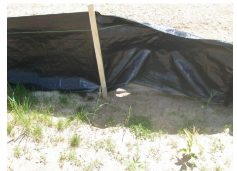
Improperly trenched silt fence
