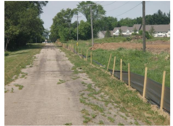
Poor silt fence install and maintenance
